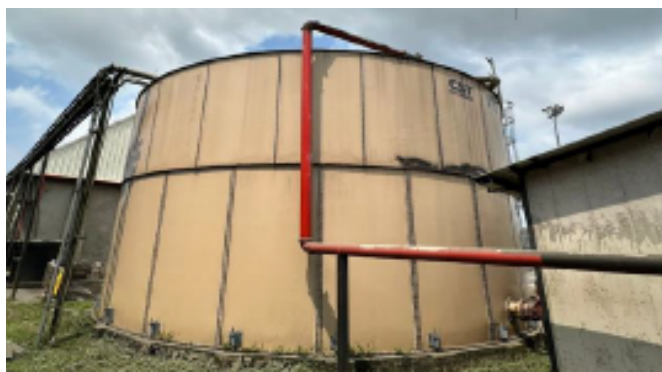
Rainwater fire fighting network storage tank 397 M 3 .
