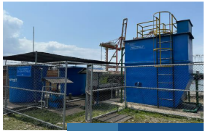
Drinking water treatment plant and treated water tank, 13 m 3 plant, and 2 tanks of 5m 3 .
